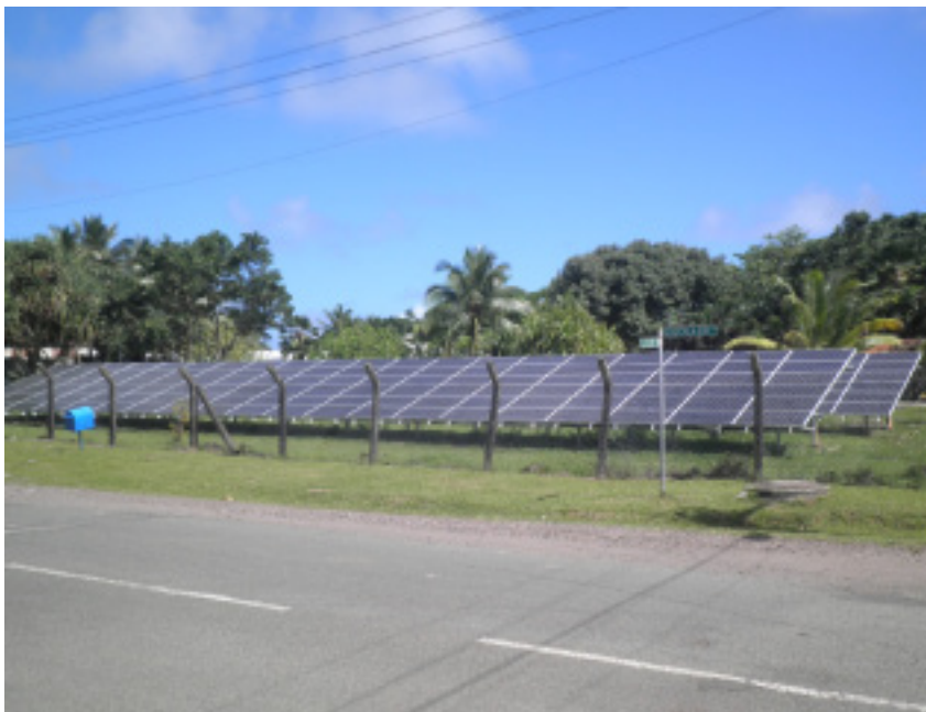
Figure 3: 45 kW grid-connected solar PV system at USP Lower Campus, Suva, Fiji Islands
