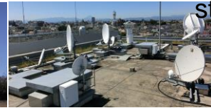
Satellite receiver antennas
