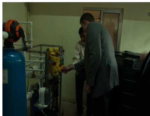
250 LPH Nanofiltration Plant installed at Jigani, Bangalore
