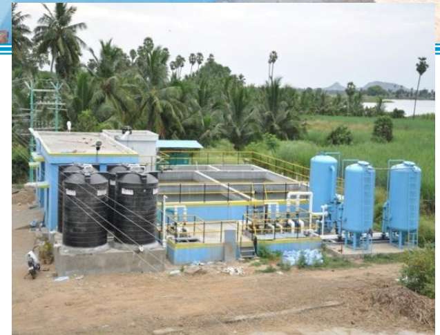
Membrane systems for water treatment
