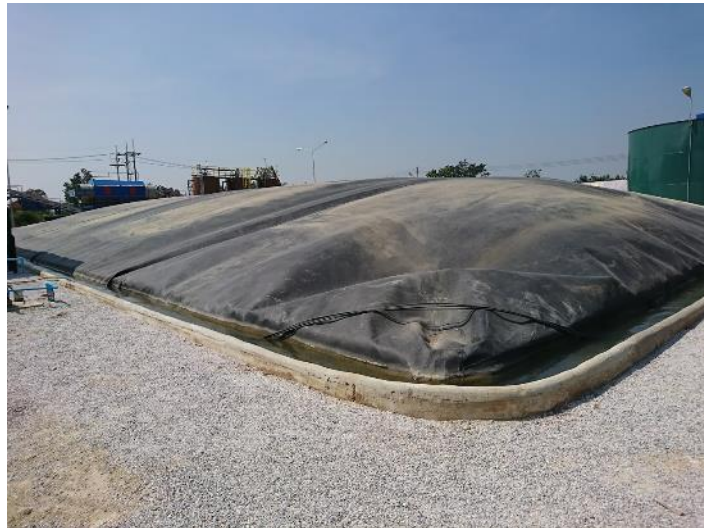
2-stage ABR (Anaerobic baffled reactor) 10 ton/day , 1,600 m 3
