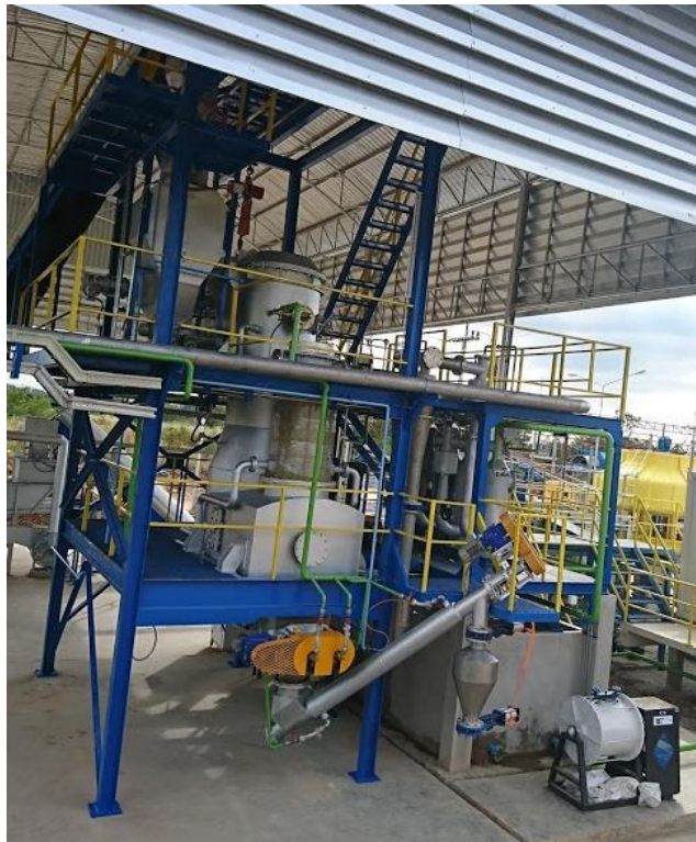
3-stage Gasification, 7.5 Ton Biomass/Day
