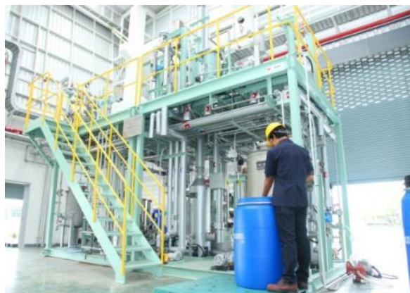
Pilot plant for biodiesel production (1000 L/day)
