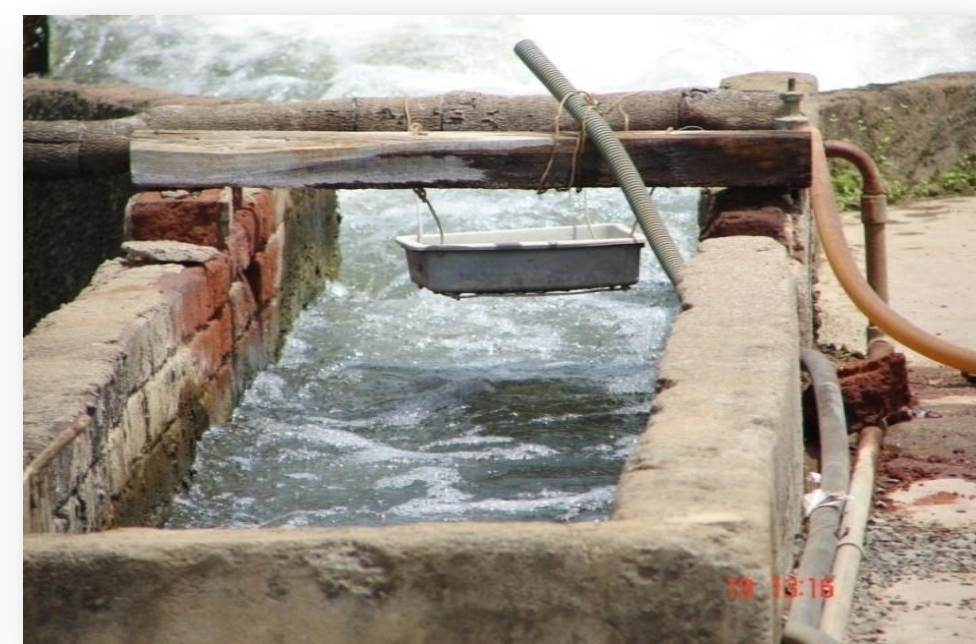
Unregulated Flow of PAC Dose at Kanhan Treatment Plant
