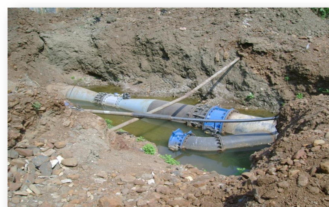
Fitting of bulk flow meters and HDPE pipes eliminates problem of pilferage
