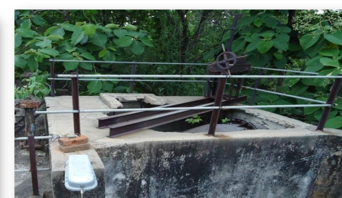
Broken Inlet Chamber of Master Balancing Reservoir at Seminary Hill
