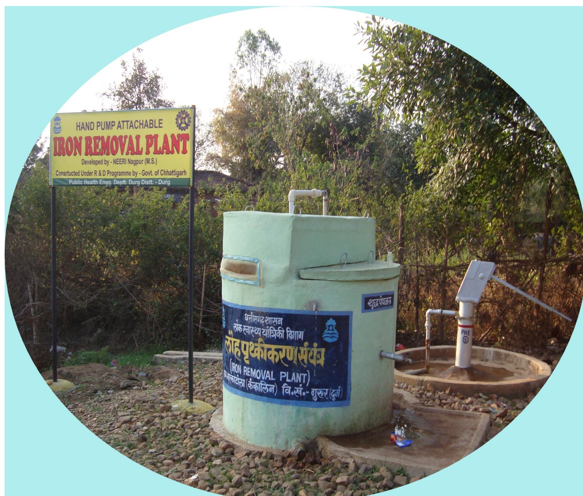
HP attachable Iron Removal Plant – RCC Structure (To be fabricated onsite)
