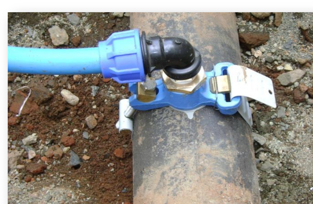
By pass valves installed at Seminary Hills MBR to facilitate cleaning and repair
