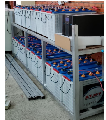
Power backup system
