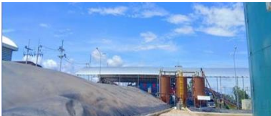
2-stage Anaerobic Baffled Reactor Biogas Production
