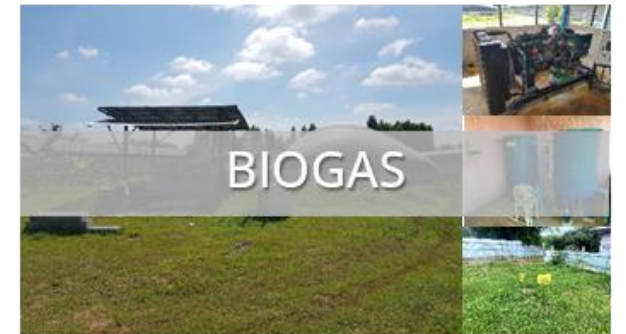
Biogas Plant + 60 kVA Generator @Ban Kham Khaen, Khon Kaen
