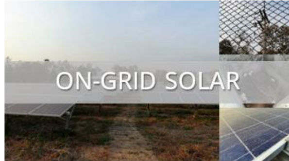
700 kW Solar Power Plant @CMRU, Chiang Mai
