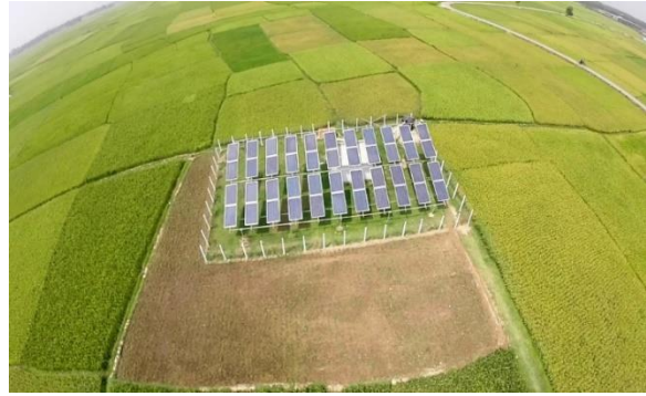
1,523 Solar Irrigation Pumps – 42 MWp
