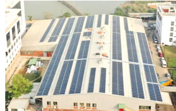
55 MWp Solar Roof top Projects
