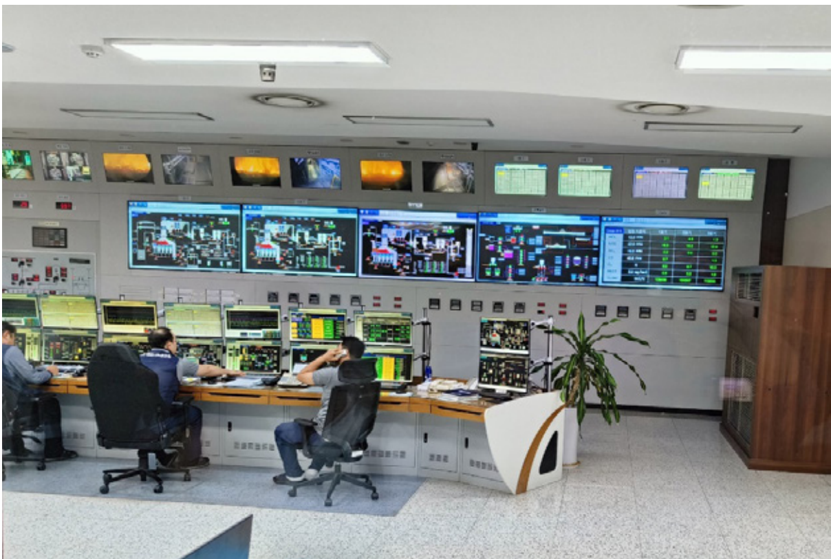
Figure 22: Waste Incineration Plant-Gangnam
